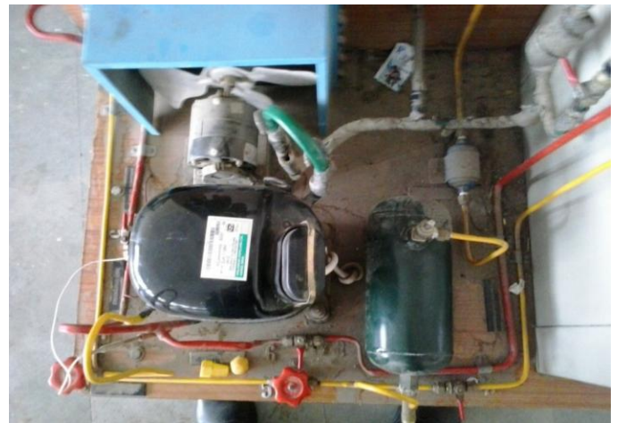
Figure 3. Ice Plant Compressor & Condenser
